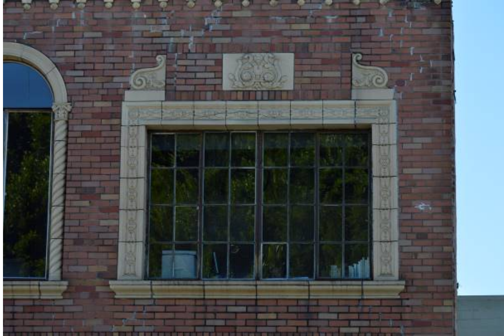
Figure 5: Fixed, steel-sash divided-light window with terracotta surround. Identical windows are located at western (shown) and eastern bay of second story, primary façade. Looking south.
