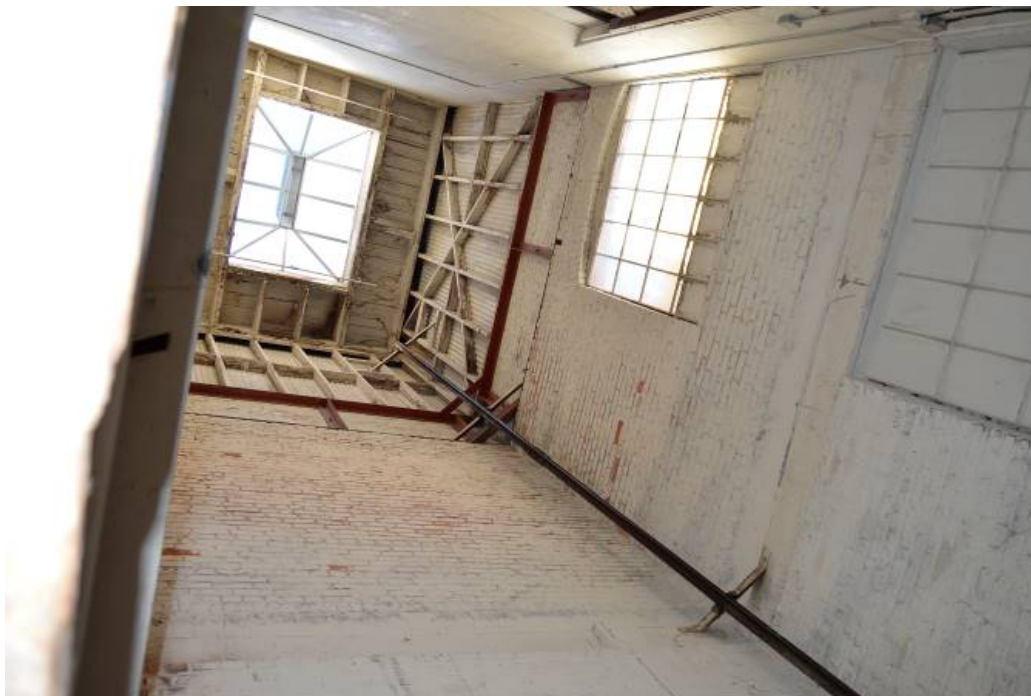
Figure 10: Interior shaft space at southeast corner of building. Second-story window at south façade picture right. Skylight at roof level pictured left. Facing south.
