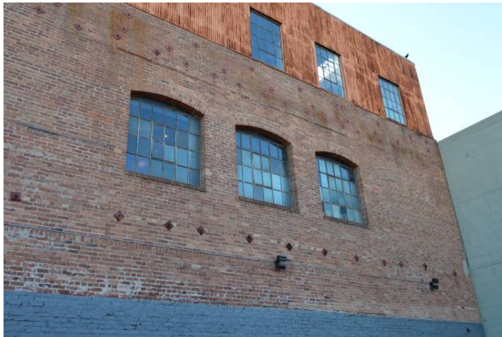
Figure 12: Steel-sash windows at second and third floors of the west façade. Looking east.
