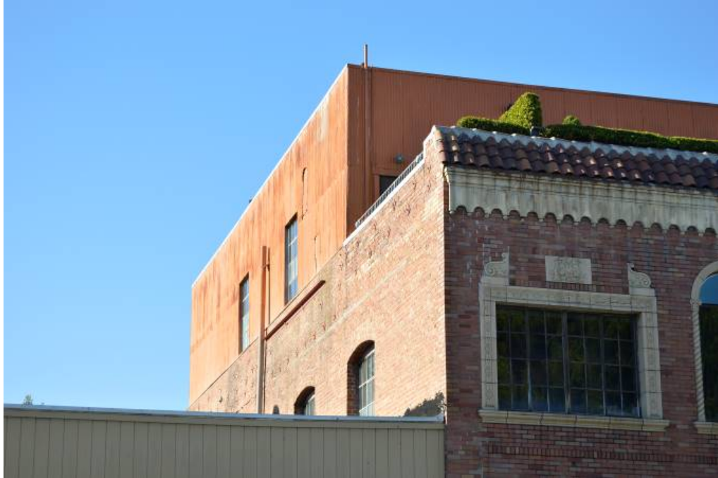
Figure 7: Second and third stories, east façade viewed from 7th Street. Looking south.
