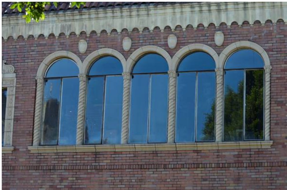
Figure 4: Grouping of five round-arched, steel-sash windows; second story, primary façade. Looking south.
